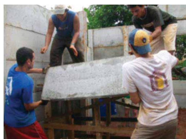
Putting up the walls was the most difficult and dangerous part. Each concrete slab weighed about 120 lbs.
