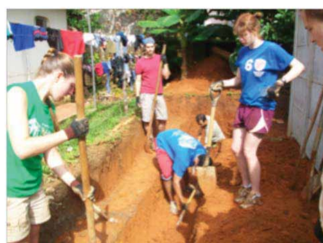
We bantered as we took turns digging the trench for the septic tank.
