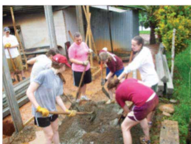
Mixing concrete was difficult, especially when all the water spilled out like a volcano and we had to scramble to put it back in.
